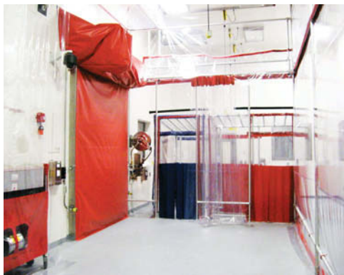
View from inside of newly installed "Biobubble" BSL-3 containment enclosure. This is actually a portable biosafety room constructed within the food processing room of the BRI, which is itself BSL-3. This gives a very high level of protection for workers conducting large studies that generate infective aerosols. (Photos courtesy of BRI)
